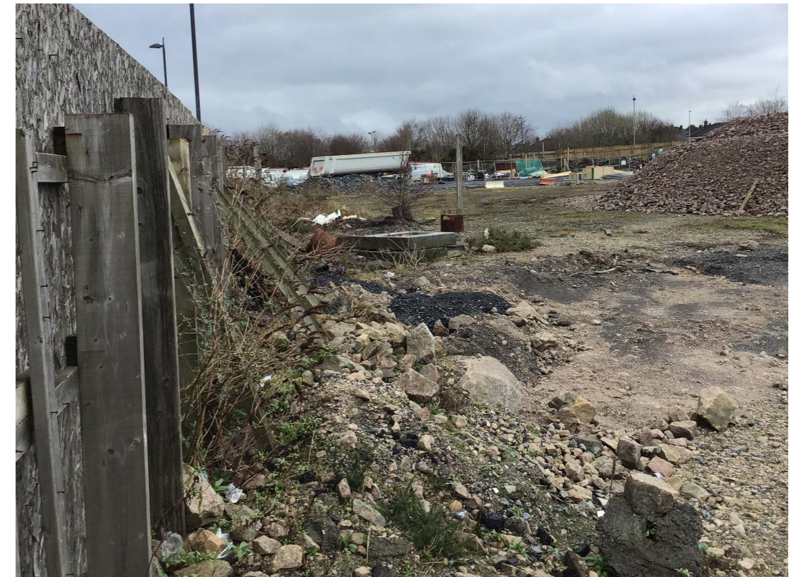
An image taken from within the site hoarding looking from the south-west to the north
